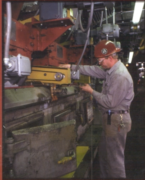
Service Representative replacing a feeder
